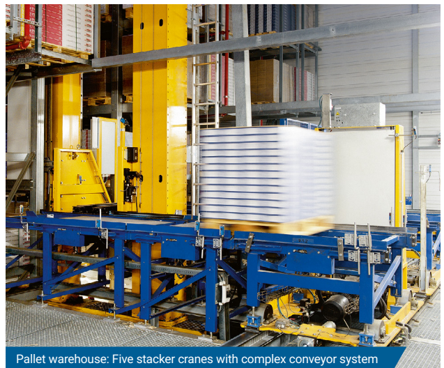
Pallet warehouse: Five stacker cranes with complex conveyor system
