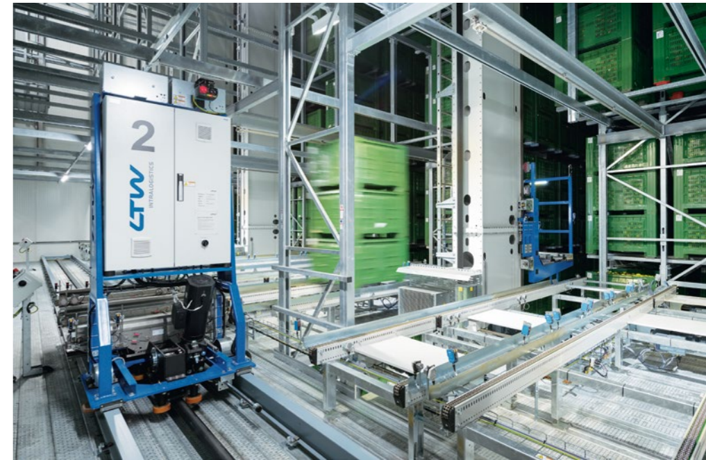
Not only the 28 meter high stacker cranes are equipped with LTW belt technology, but also the two transfer cars in the pre-zone (image) and two vertical conveyors. The non-slip drive and the absolute length constancy of the belt allow high kinematic values and minimum settling times.
