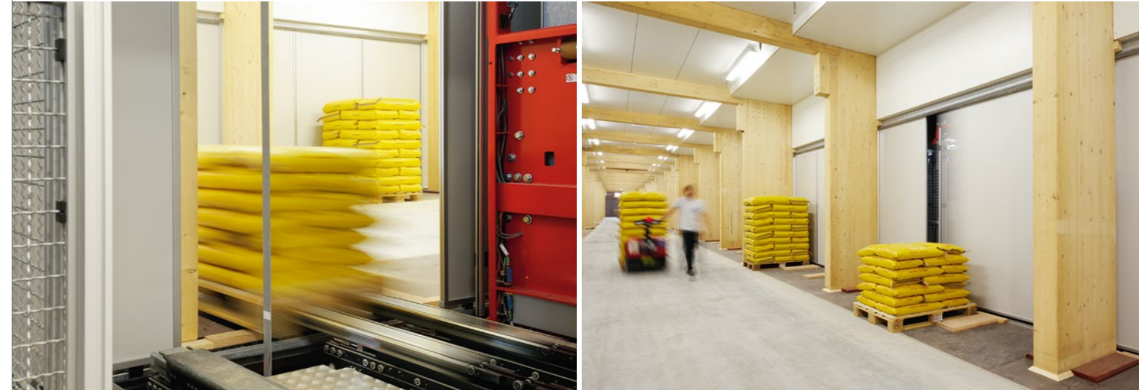
Four stacker cranes supply from both sides three spacious and well-lit order picking tunnels that range over the entire length of the high-bay warehouse. 324 order picking gates by LTW provide safe separation between the tunnel and the stacker crane aisles as required by safety regulations.
