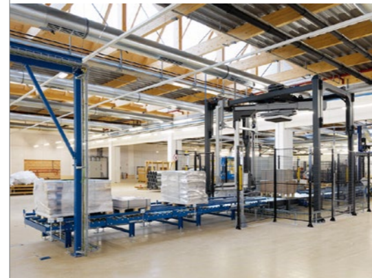
Conveyor line with automatic contour control, strapping, wrapping and labelling for pallets of different dimensions.
