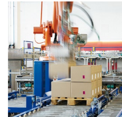
The existing robot was integrated into the new fully-automatic cardboard box conveying equipment with precise timing and minimum service interruption.
