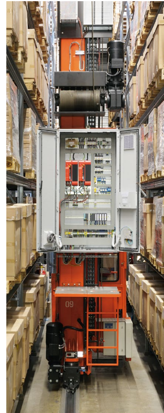
After just three days of conversion work and testing this storage and retrieval machine, which now has a S7-switch cabinet and new driving and hoisting drives, was again ready for immediate use.
