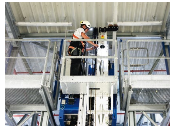
Even when designing the high-bay warehouse, safe and ergonomic work must be provided for service, e.g. with rugged maintenance cages on the rack.
