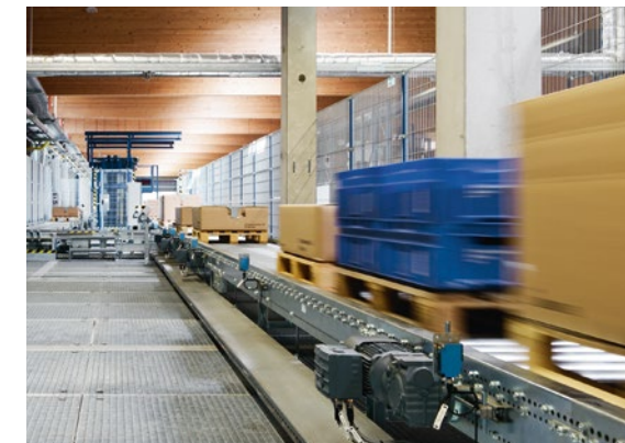
As general contractor for intralogistics LTW maintains all trades – the correspondent transfer of knowledge also takes place in the cooperation with sub-suppliers.
