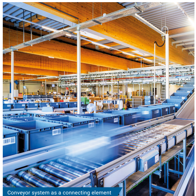
Conveyor system as a connecting element
